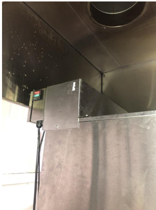
Appliance Exhaust Outlet Under Collection Hood
